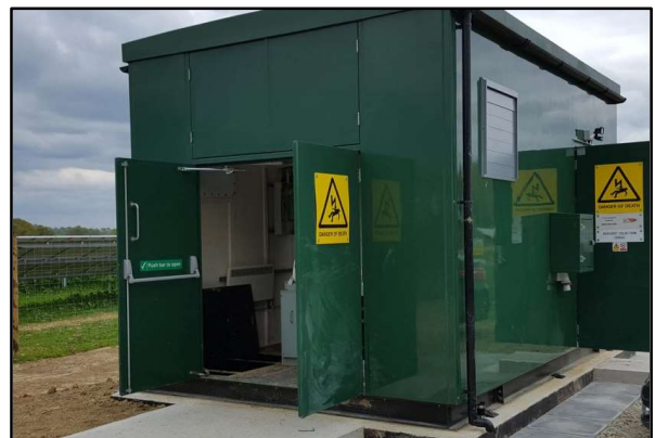
Example Transformer Unit on site
